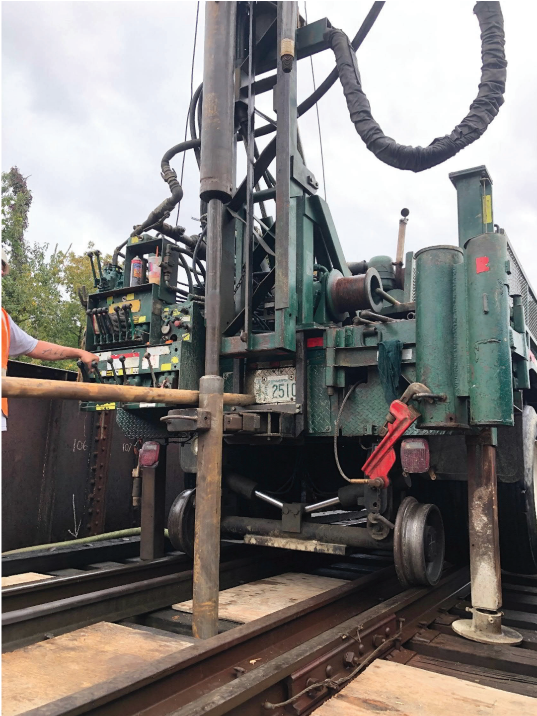
Figure B2: Boring B-2 Drilling (on the east side of the Center Pier)
