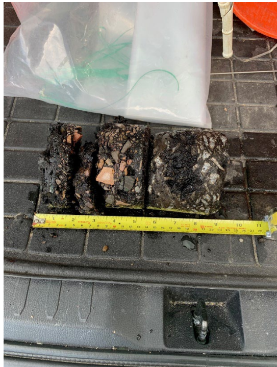
Asphalt core extracted at MM 58.0, Right Lane
