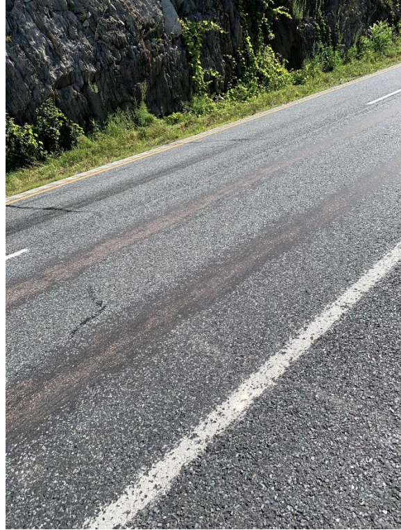
Surface Distresses at MM 61.0, Right Lane
