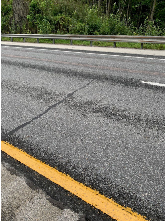
Surface Distresses at MM 61.0, Left Lane
