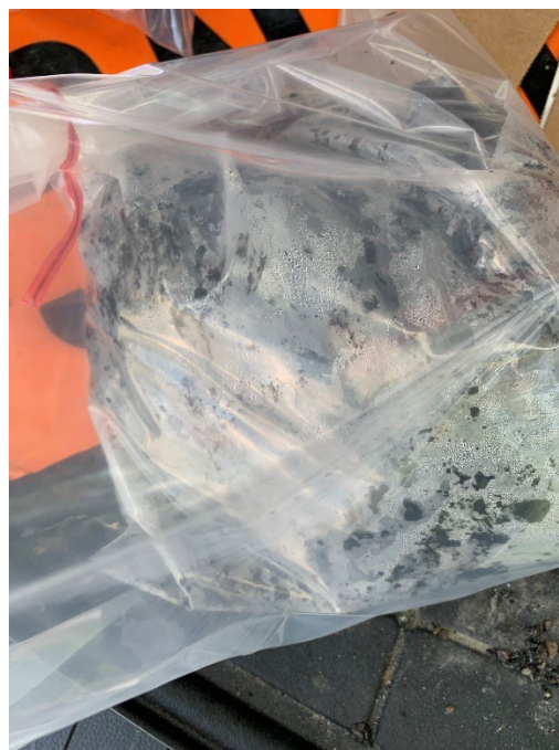
Asphalt core extracted at MM 52.85, Right Lane. The core completely disintegrated when extracted.
