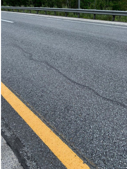
Surface Distresses at MM 54.0, Left Lane
