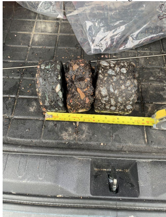
Asphalt core extracted at MM 57.0, Right Lane.
