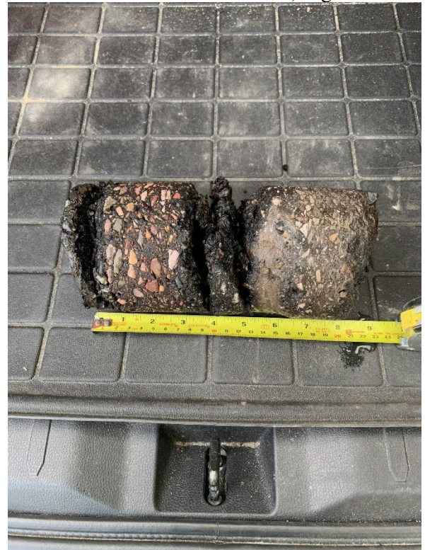
Asphalt core extracted at MM 62.0, Right Lane
