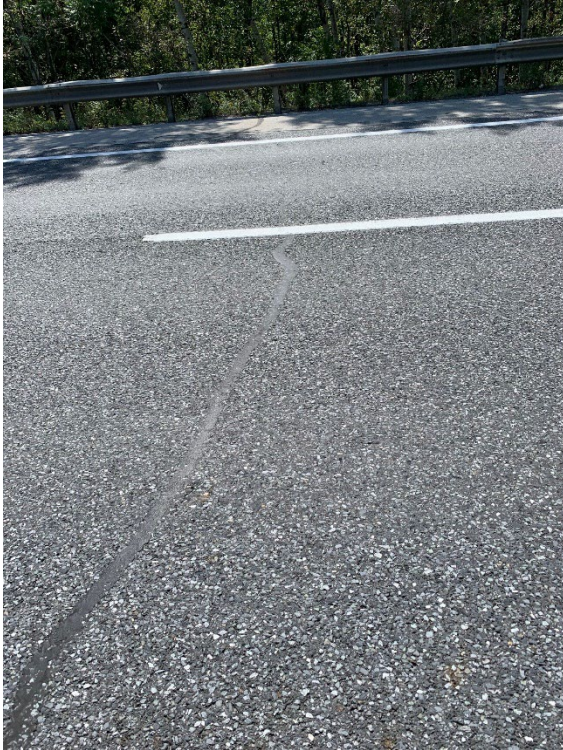
Surface Distresses at MM 60.0, Left Lane
