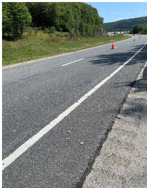
Surface Distresses at MM 52.85, Right Lane
