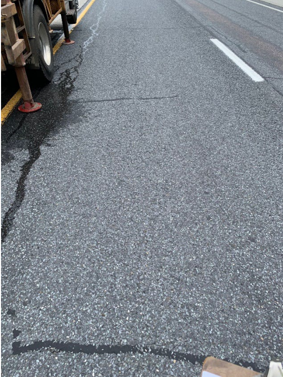
Surface Distresses at MM 58.0, Left Lane
