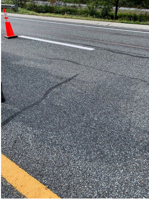
Surface Distresses at MM 55.0, Left Lane
