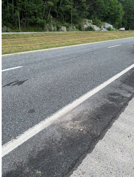
Surface Distresses at MM 57.0, Right Lane
