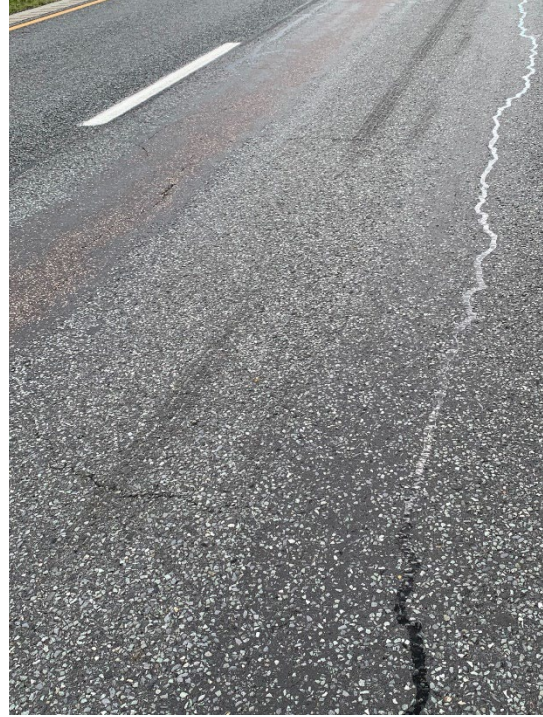
Surface Distresses at MM 58.0, Right Lane
