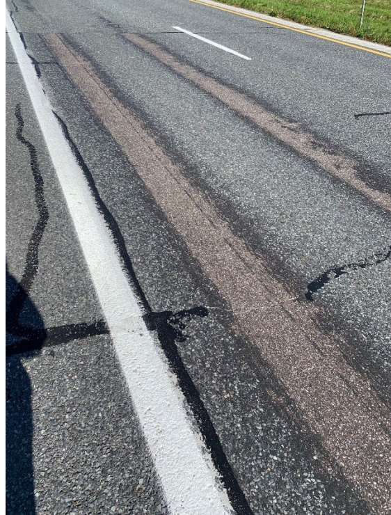
Surface Distresses at MM 60.0, Right Lane
