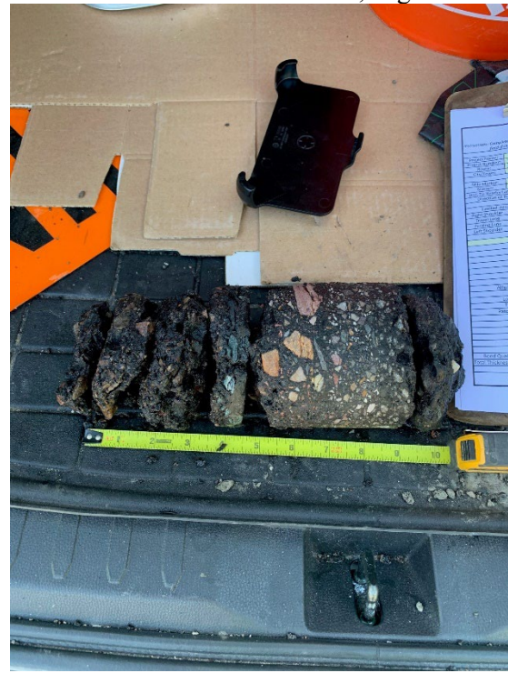
Asphalt core extracted at MM 60.0, Right Lane
