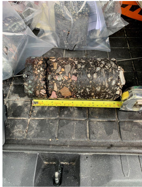
Asphalt core extracted at MM 55.0, Right Lane
