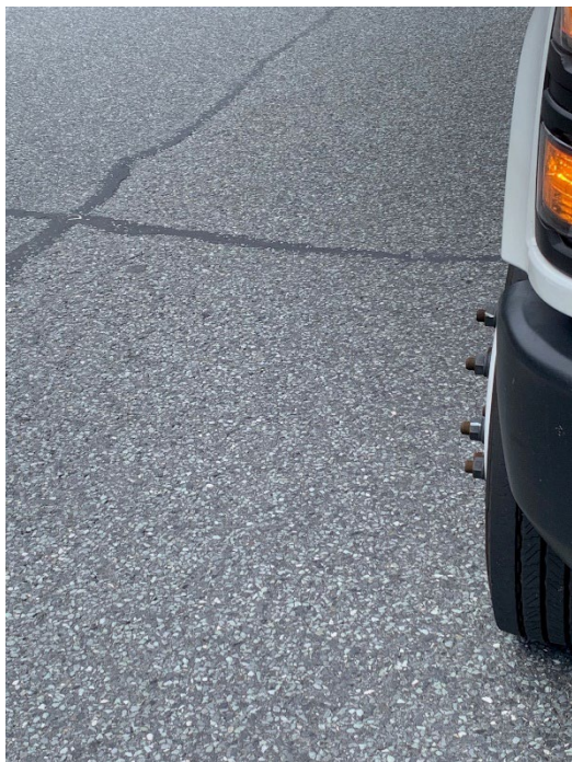
Surface Distresses at MM 52.85, Left Lane; photograph taken in front of drilling rig.
