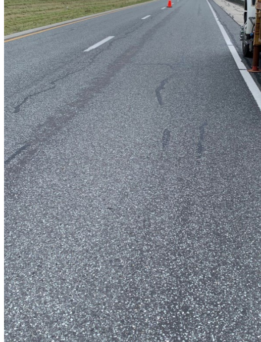
Surface Distresses at MM 54.0, Right Lane
