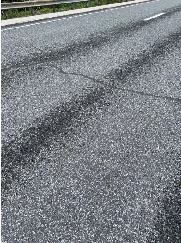
Surface Distresses at MM 59.05, Left Lane
