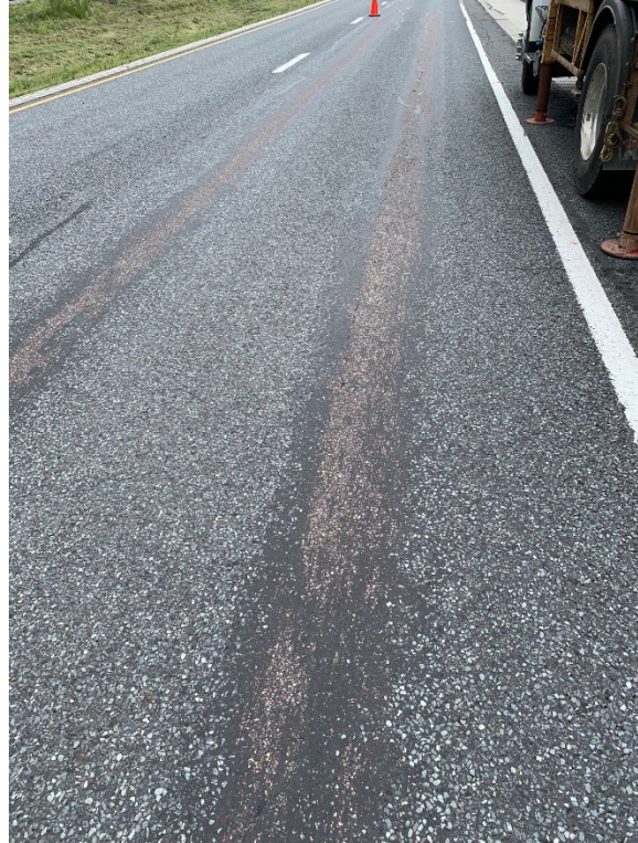
Surface Distresses at MM 55.0, Right Lane
