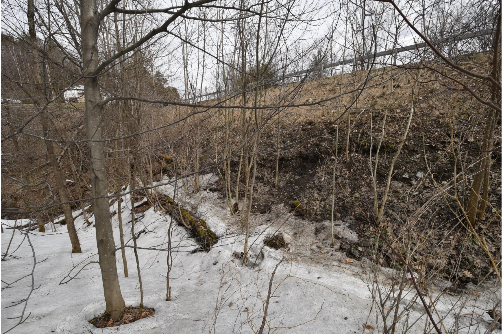
Figure 4: MM 6.28 Surficial Failure at Toe of Slope
